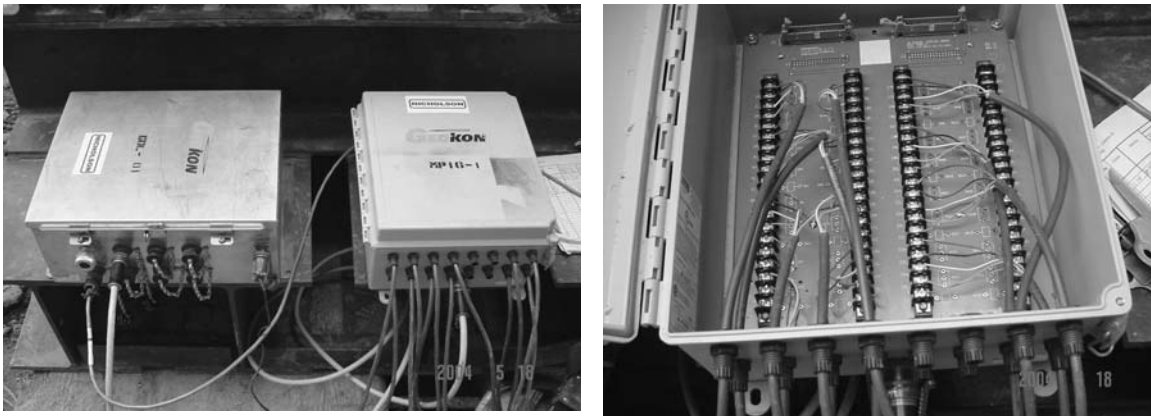
Figure 2 Datalogger and Multiplexer
