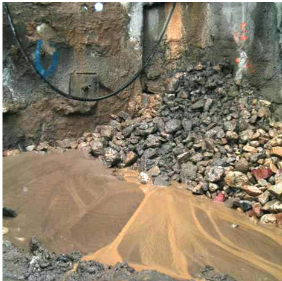
Figure 10. Seepage inflow at the connection between the diaphragm wall and the jet grout cutoff.
