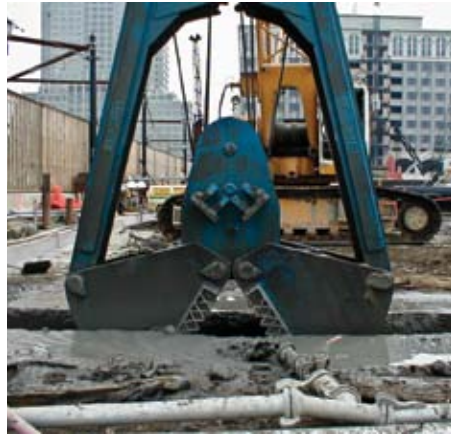
Anchor installation through diaphragm wall (left) Diaphragm wall excavation with clamshell (right)
